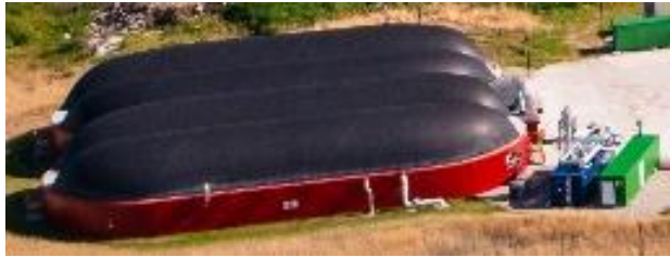
Biodigester, located on the Goodrich Family Farm, Salisbury, VT.
